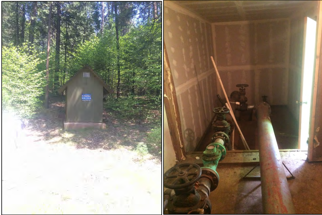
Figure 3.7a Cypress Point Booster Pump Station
